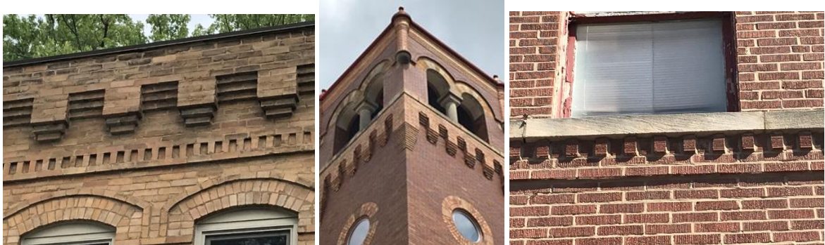
This brick was not meant to be painted
