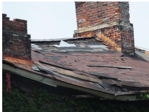
Deteriorated, Loose & Missing Shingles
