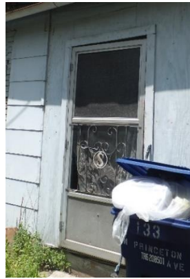
Poorly Fitted Storm Door
