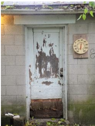
Exposed & Deteriorated Wood Door
