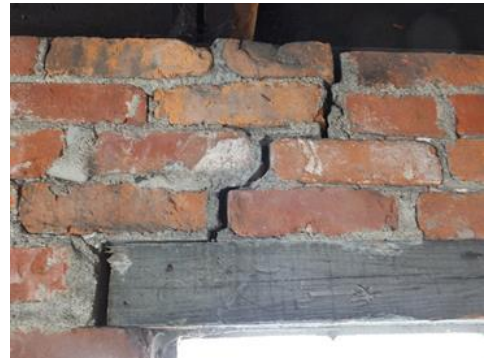
Diagonal Crack in Exterior Masonry Wall
