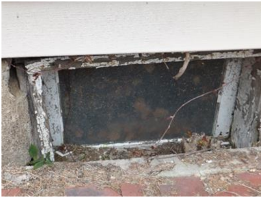
Moisture Damage, Basement Window Well
