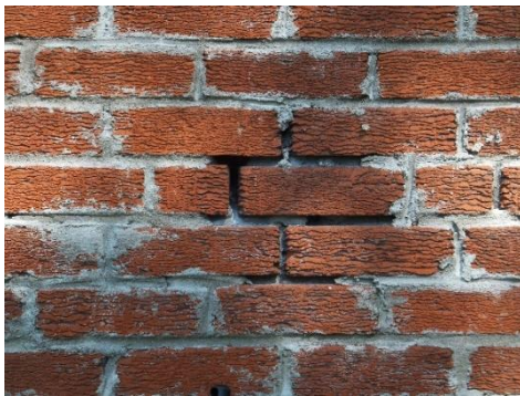
Poor Tuckpointing & Missing Mortar Joints
