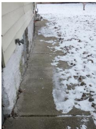
Sidewalk Sloped Toward Foundation
