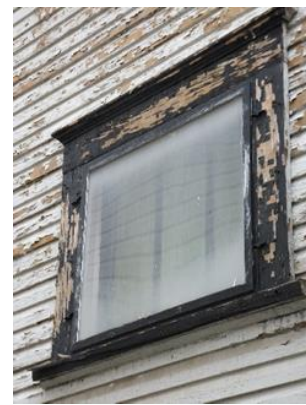
Deteriorated Storm Window
