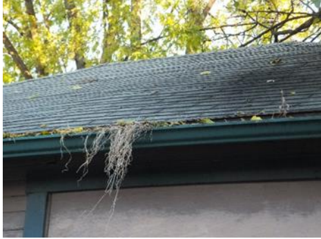
Stopped-up, Clogged Gutters
