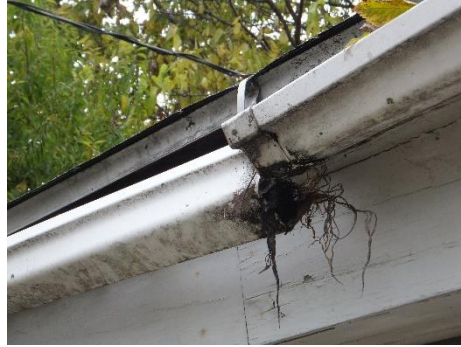
Broken Gutter Connections
