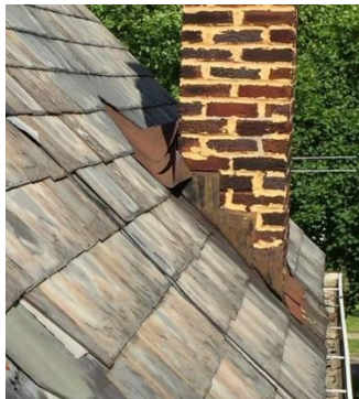
Damaged Chimney Flashing
