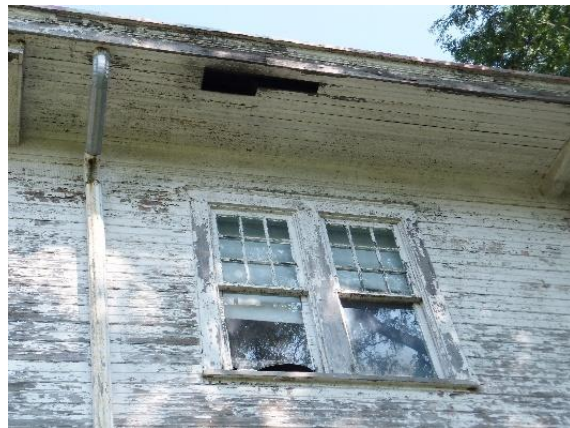
Deteriorated Paint on Siding & Windows; Soffits with Wood Rot
