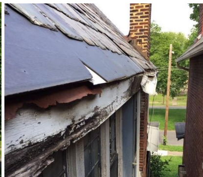
No Flashing at Roof Eaves
