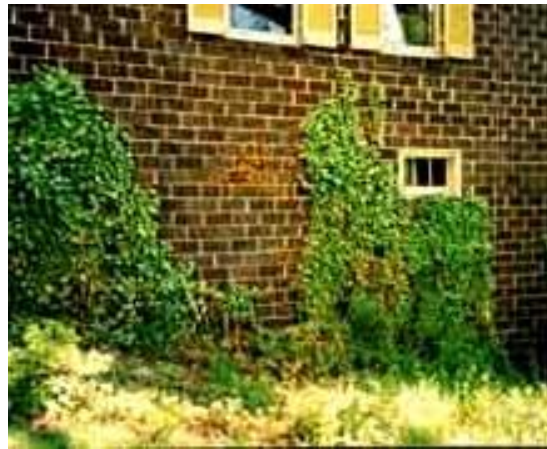
Vines Anchored to Brick Wall & Mortar Joints
